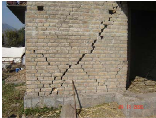
Photo 9: Diagonal cracking of solid wall (Bed joint sliding mode)
