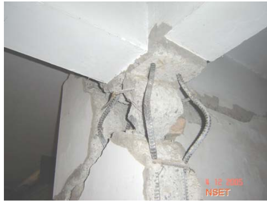
Photo 22: Buckling of column bars
