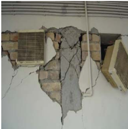
Photo 21: Shear crack in column
