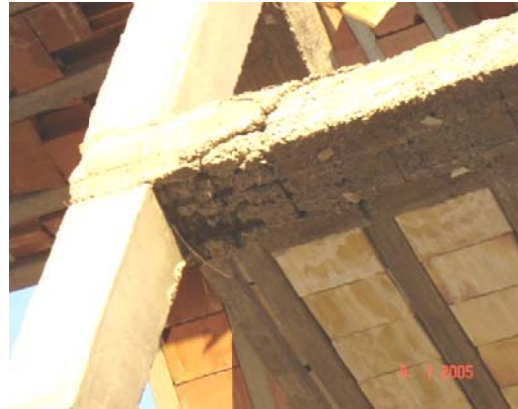
Photo 20: Shear crack in beam near to support
