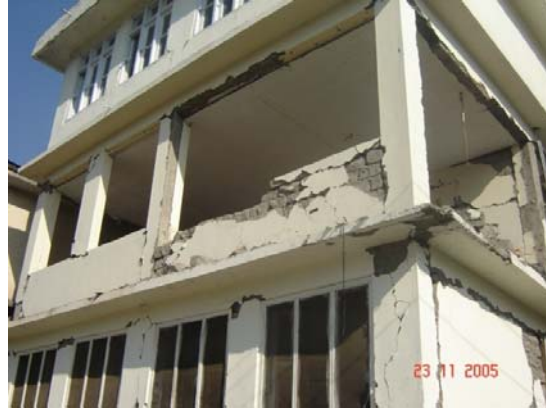
Photo 24: Extreme Damage to Infill wall
