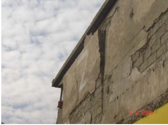
Photo 23: Moderate-Heavy Damage to Infill wall
