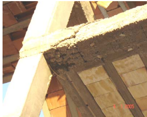
Photo 20: Shear crack in beam near to support
