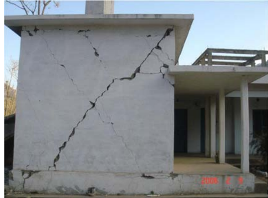
Photo 8: Diagonal cracking of solid wall
