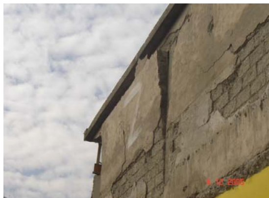
Photo 23: Moderate-Heavy Damage to Infill wall
