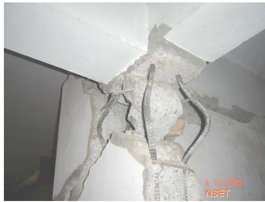
Photo 22: Buckling of column bars
