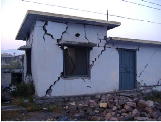
Photo7: Diagonal cracking of masonry piers starting from corner of openings
