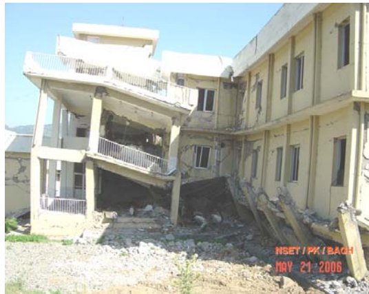
Photo 18: Earthquake damage due to soft story
