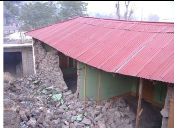
Photo 10: Out of plane failure of stone wall
