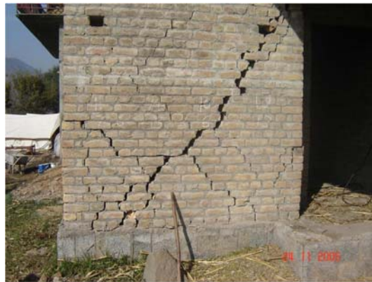
Photo 9: Diagonal cracking of solid wall (Bed joint sliding mode)
