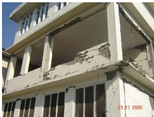
Photo 24: Extreme Damage to Infill wall
