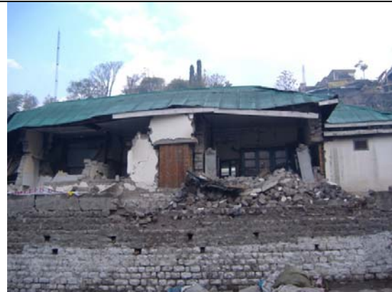
Photo 11: Out of plane failure of block wall
