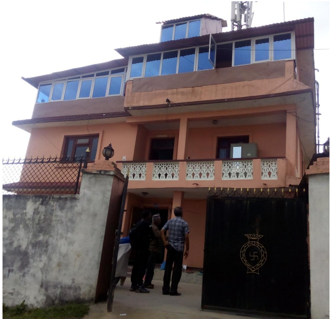
Wall bearing Structure, Kapan3 (Totally damage)
